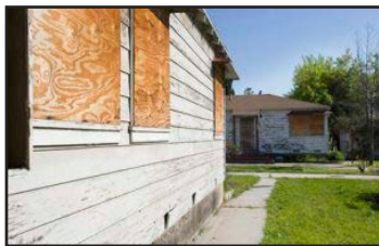
Figure 7-39 Residential home as a Board-Up Structure
