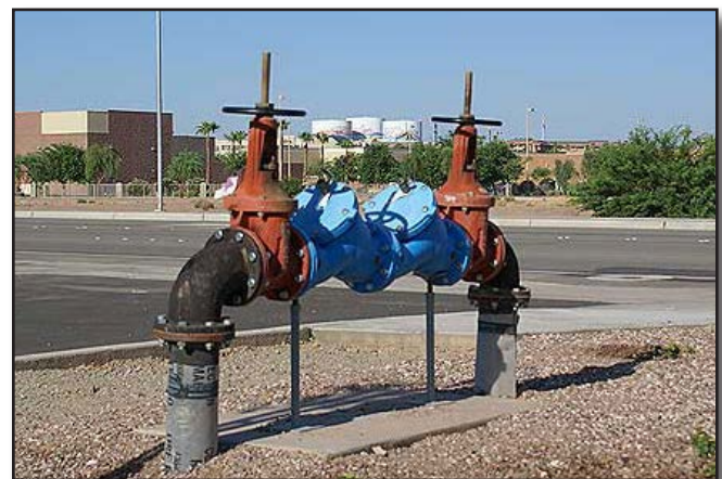
Figure 11-35 Main Water Control Valve from Municipal Water Supply with OS&Y Valves
