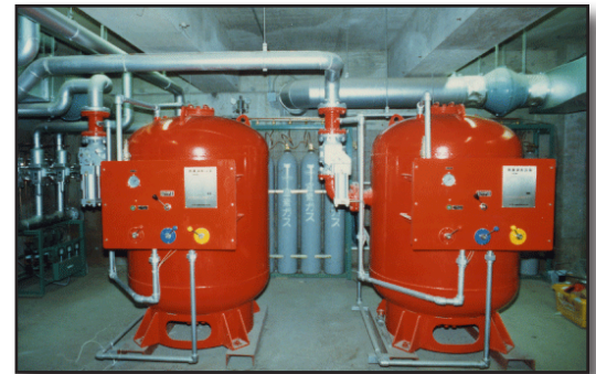
Figure 11-50 Dry Chemical System Storage Tanks
