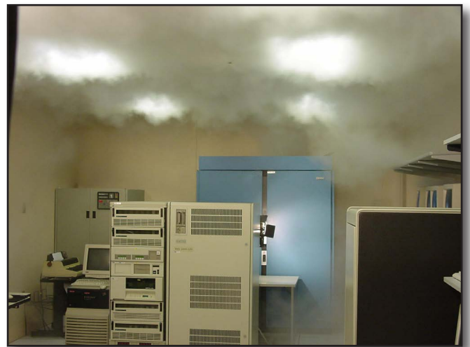
Figure 11-47 Halon Extinguishing System
