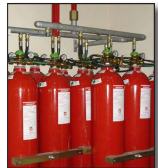
Figure 11-48 Halon Storage System
