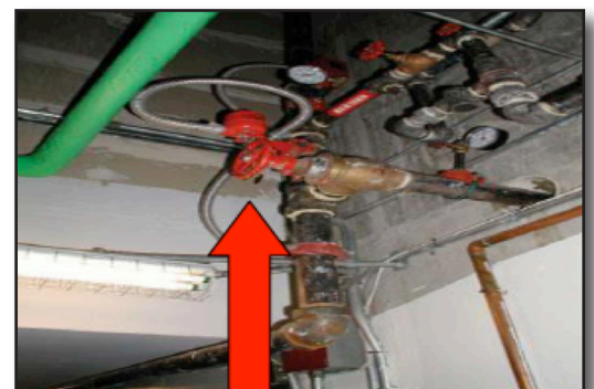
Figure 11-45 Zone/Floor Control Valve Located Overhead in the Plenum Space
