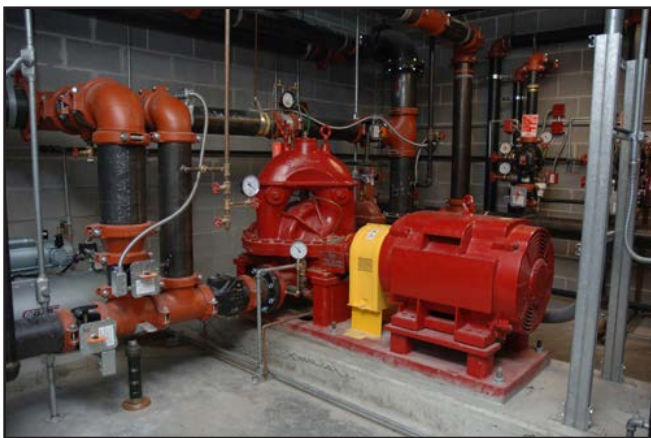
Figure 11-42 Fire Protection System Pump
