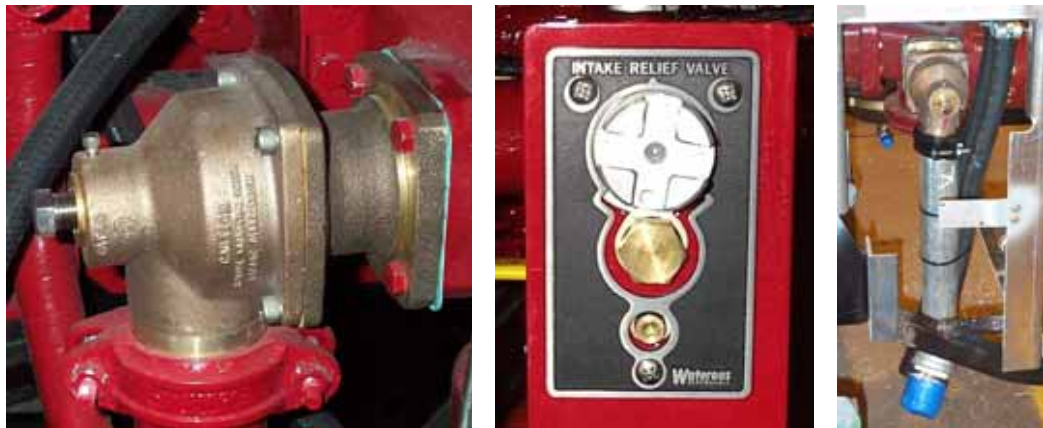
Figure 2-1: Typical Intake Relief Valve ( relief outlet pipe with threaded end shown on right )
