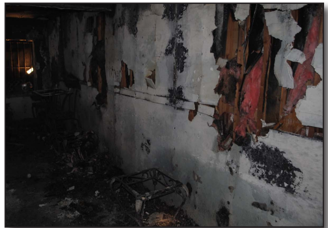
Figure 33-12 A good example of systematic overhaul with minimal damage prior to the investigators arrival
