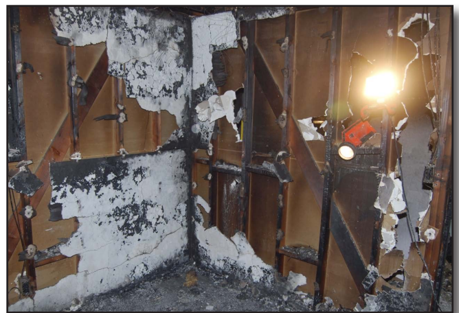
Figure 33-13 Excessive overhaul prior to the investigators arrival can destroy the scene and fire patterns.
