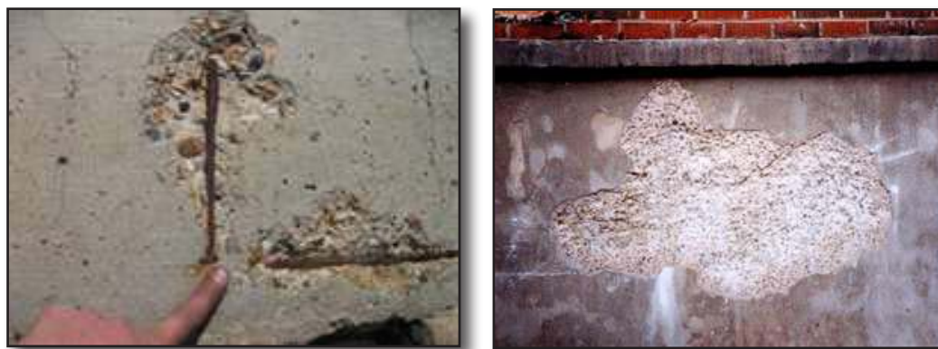
Figure 33-7 Spalling (above 2 images)
