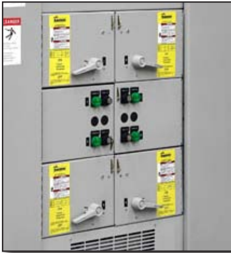
Figure 32-19 Typical Main Power Disconnect in Elevator Machine Room
