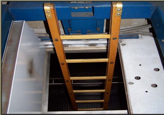
A pole ladder can then be placed into the elevator cab for extraction of passengers
