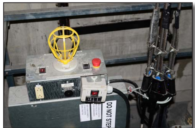
Figure 32-13 Inspection Station (top of elevator car)
