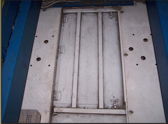
Top view of emergency escape hatch on elevator cab.
