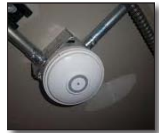
Figure 32-2 FAID found in Elevator Machine Room
