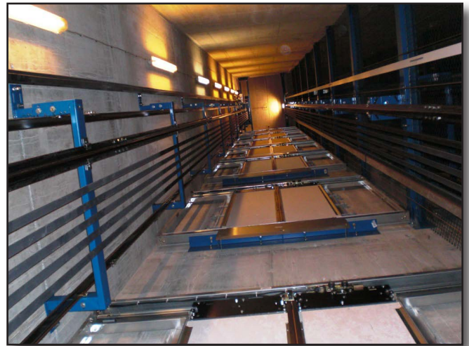
Figure 32-7 Common Elevator Hoistway
