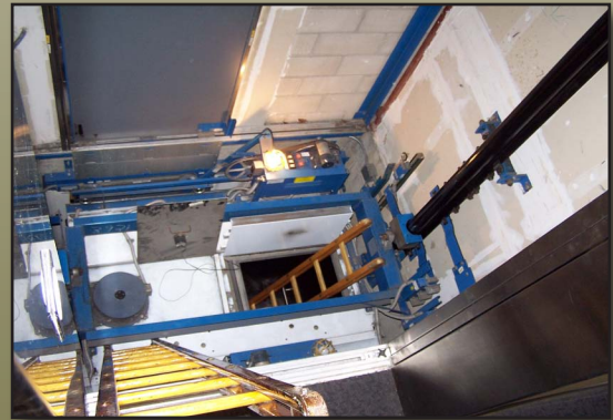
A second ladder may be used to assist passengers and rescuers climb out of the elevator shaft
