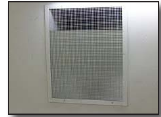
Figure 31-32 Stairwell pressurization vent
