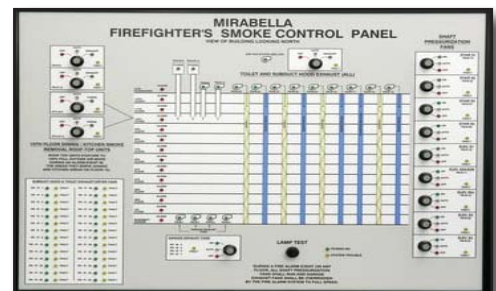
Figure 31-41 Smoke Handling & Pressurization System Panel located in Fire Control Room
