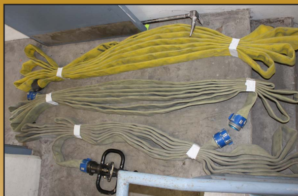
Lay out the hose packs on the fire floor landing aligning the couplings & attach nozzle
