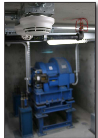
Figure 31-49 An activated Fire Alarm Initiating Device (FAID) inside of the elevator machine room will send the elevators into Automatic Phase I Recall - Do Not Use!
