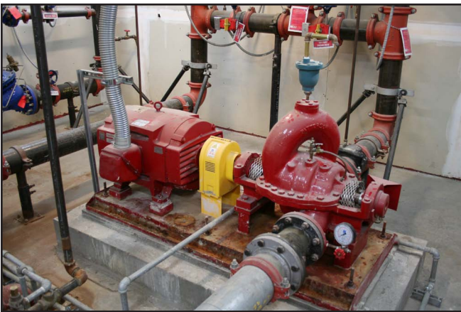
Figure 31-52 A typical building fire pump
