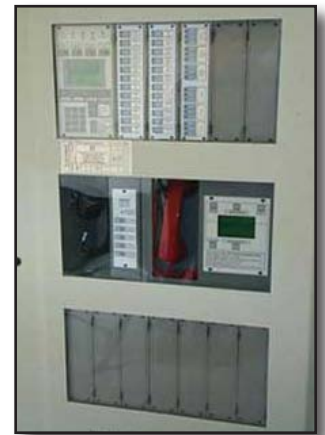
Figure 31-16 Typical High-Rise Alarm Panel
