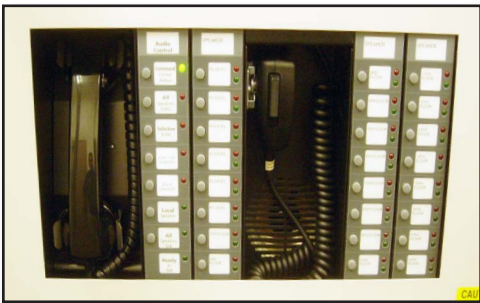
Figure 31-44 Public Address System (often incorporated into the alarm panel)
