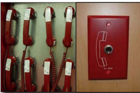
Figure 31-45 Interior communication system (Red Phones)
