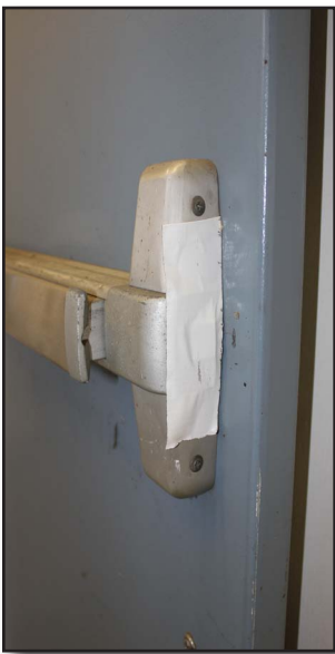
Figure 31-34 Duct tape placed over the door latch allows the door to close for stairwell pressurization but not lock you out
