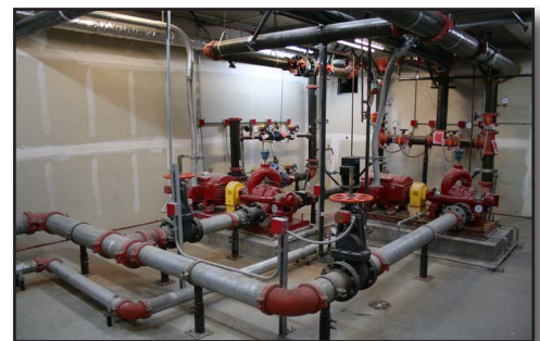
Figure 31-42 Building Fire Pump
