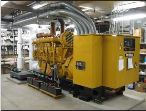
Figure 31-43 Power Generators may be found in certain modern high-rise buildings
