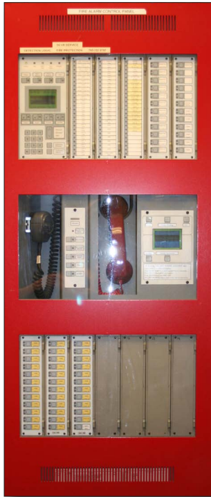
Figure 31-38 Fire Alarm / Annunciator Panel
