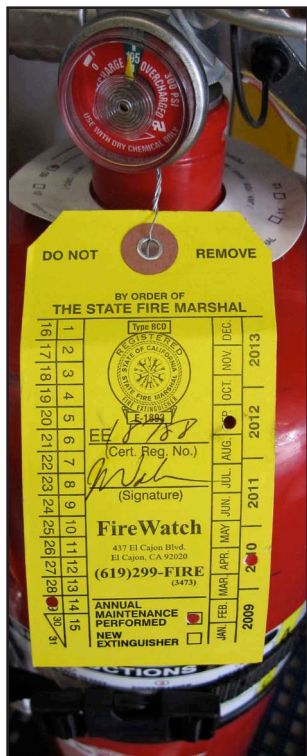
Figure 10-10 Fire ext. service tag
