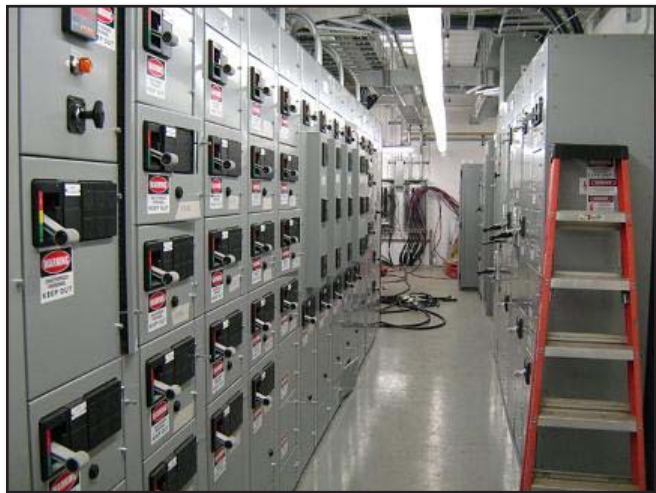
Figure 10-5 Halogenated agents are ideal for extinguishing fires in electrical and computer equipment rooms
