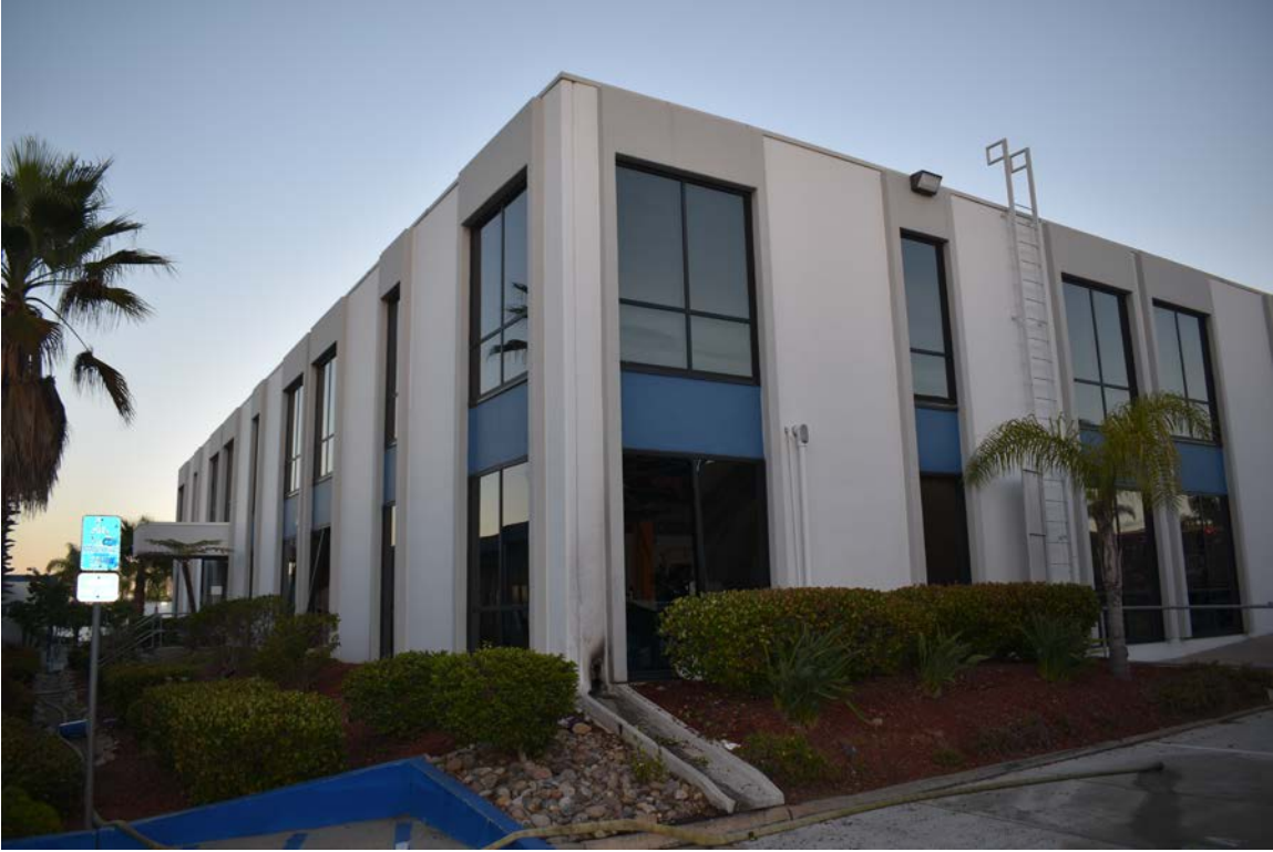
Photo No. 3: Bravo – Charlie corner. Smoke damage from bottom drains.
