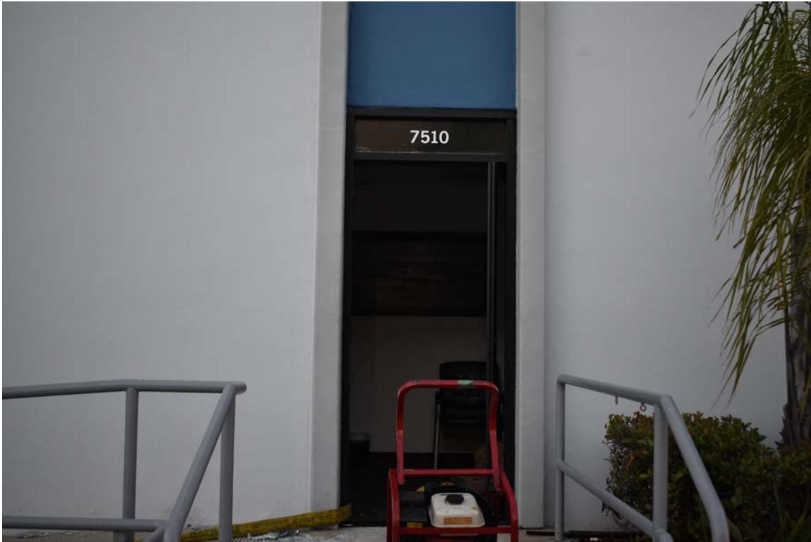
Photo No. 7: Forced door.
