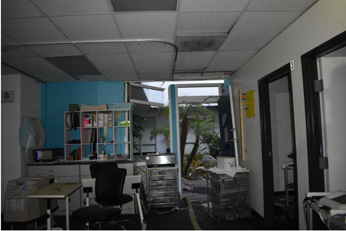
Photo No. 9: Access door to center courtyard. High level severe structural damage.
