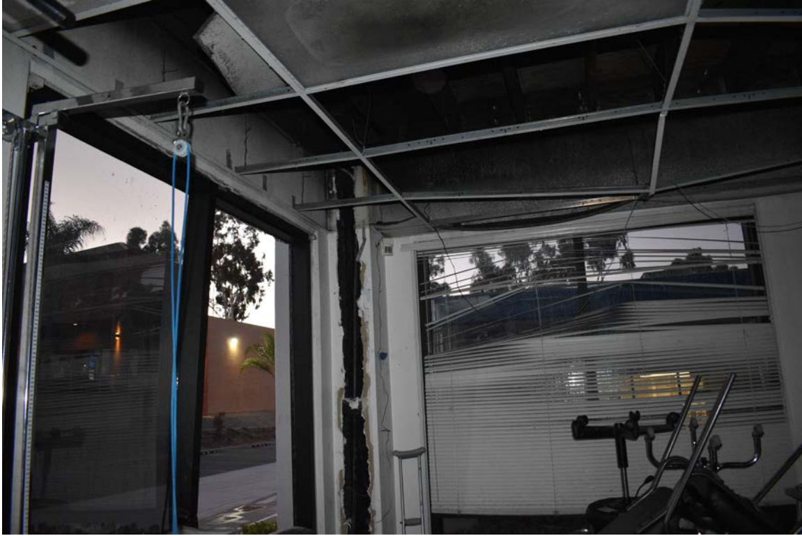
Photo No. 11: Alpha – Bravo corner; area of origin of fire. ABS pipe and electrical conduit present.
