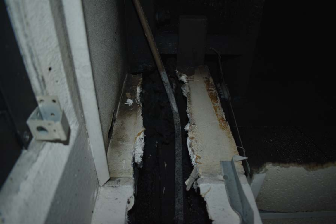
Photo No. 13: Perforation in chase allowing for conduit passage and exhausting of combustion gas
