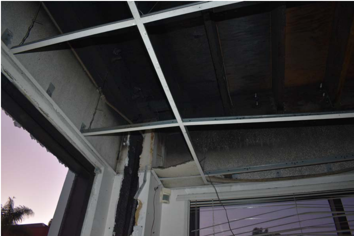
Photo No. 12: Localized smoke staining to plenum between T-bar panels and ceiling.
