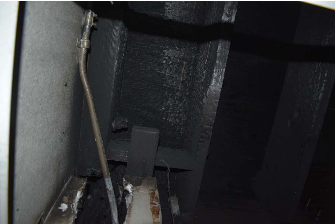
Photo No. 14: Ceiling – Floor Joists above area of origin. Location of escaping combustion gases.
