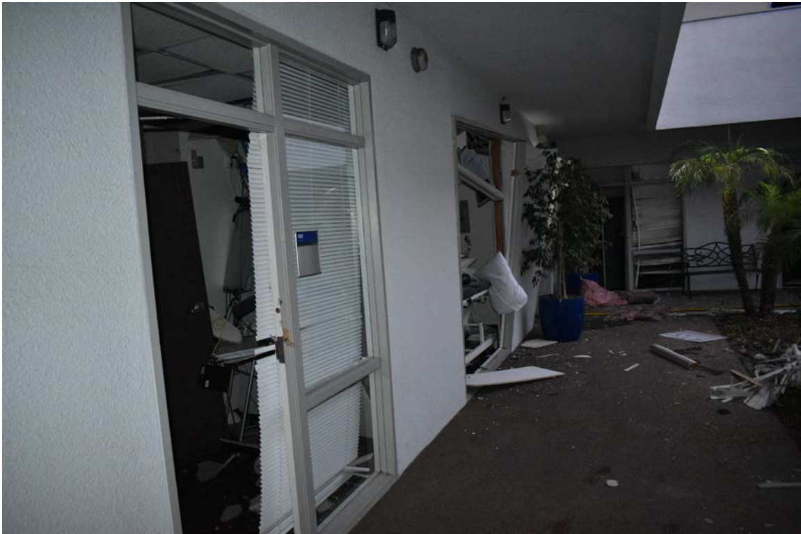
Photo No. 10: Protruding door and window frames; view from center courtyard.
