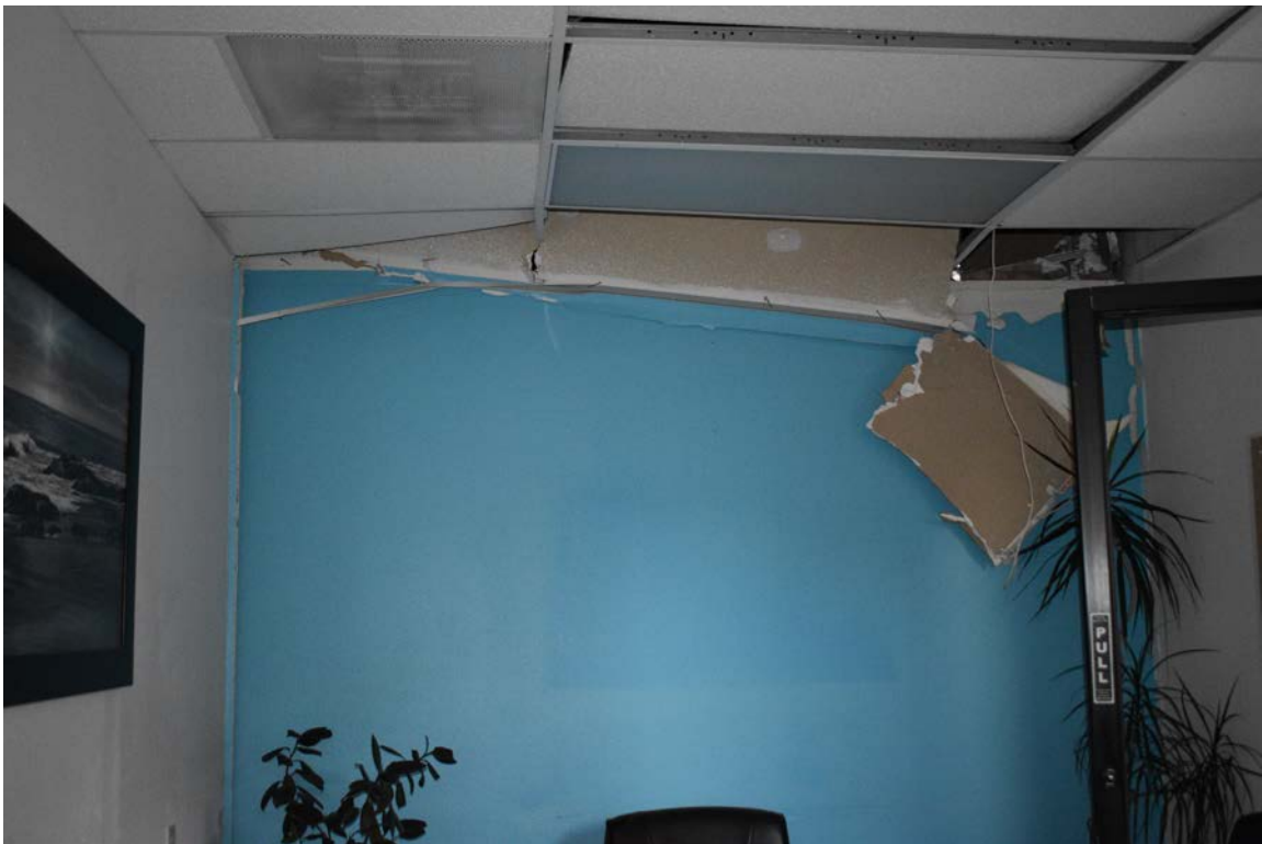
Photo No. 8: High level blast pressure structural damage.
