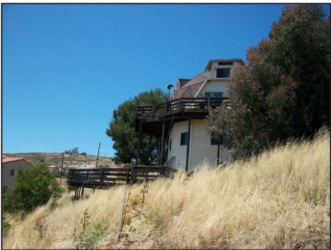
Figure 13-45 Threatened Non-Defensible: No clearing around structure, grass next to house and below wood deck, large trees close to house, house is midslope.
