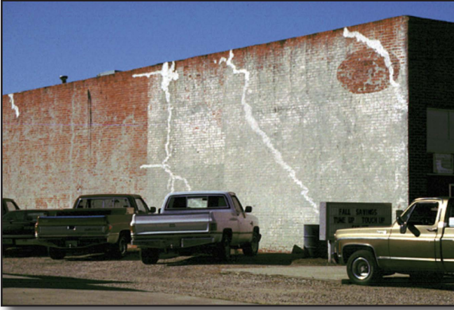
Figure 8-51 Signs of a weakened structure and potential building collapse
