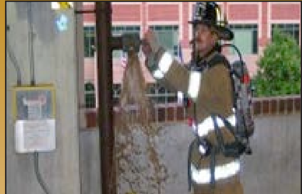
Open the standpipe valve to flush any debris and check for water flow
