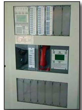
Figure 31-16 Typical High-Rise Alarm Panel
