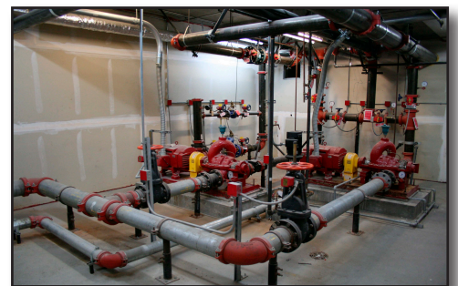
Figure 31-42 Building Fire Pump
