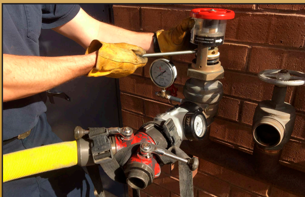
Charge hoseline and adjust PRV as necessary based upon the pressure reading from the in-line pressure gauge with water flowing.
