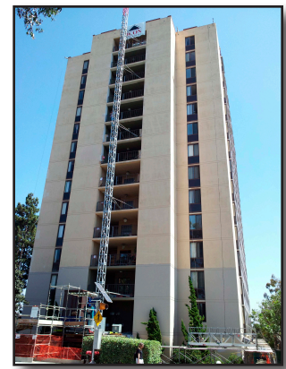
Figure 31-6 Smoke Tower with outside vestibule
