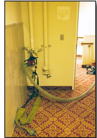
Figure 31-19 Hose lines should be connected to the standpipe 1 floor below the fire floor
