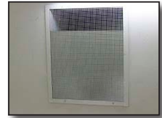
Figure 31-32 Stairwell pressurization vent
