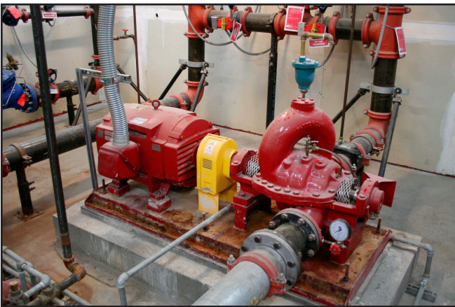
Figure 31-52 A typical building fire pump
