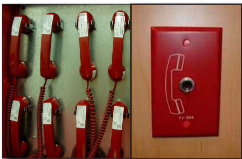
Figure 31-45 Interior communication system (Red Phones)
