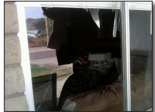
Figure 21-51 Broken Plate Glass
