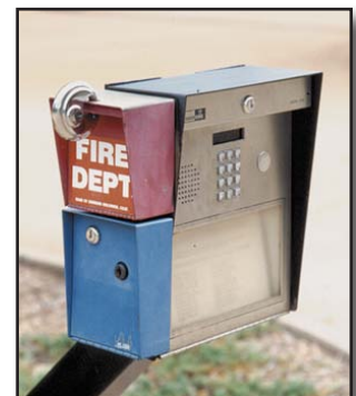
Figure 21-45 Security gate access with knox box key
