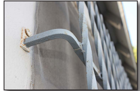
Figure 21-61 Security bars anchored into structure with a lag bolt.
