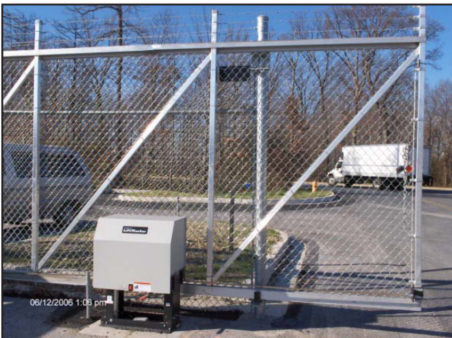
Figure 21-49 Rolling metal security gate
