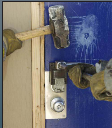
Place Adz of Halligan Bar into K-Tool then strike with sledge or axe
