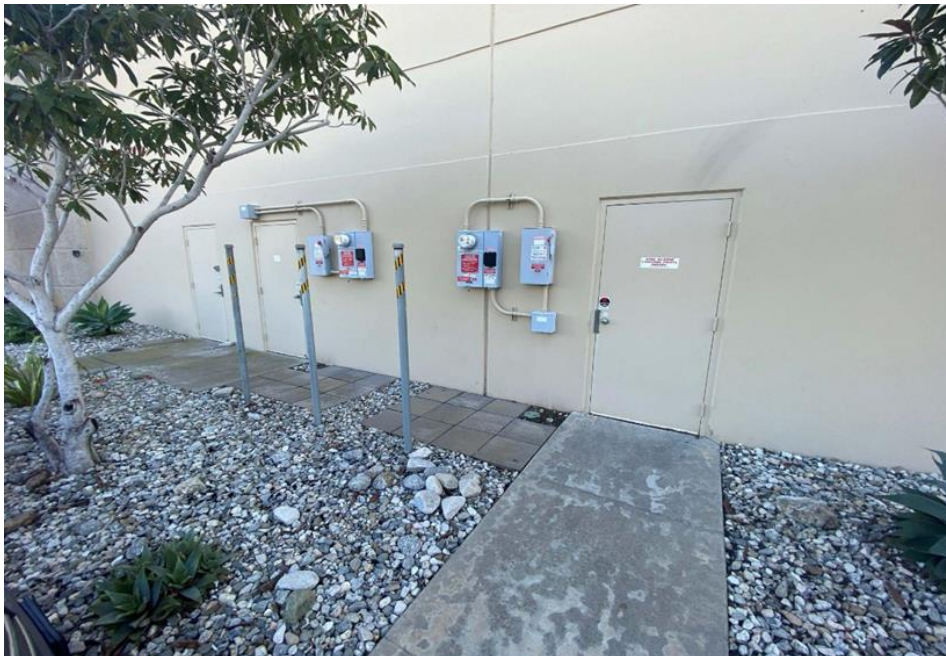
Image 4 - Electrical Room Entrances with Solar (PV) Meters and Shut Offs
