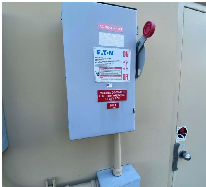
Image 6 - Solar (PV) Disconnect
