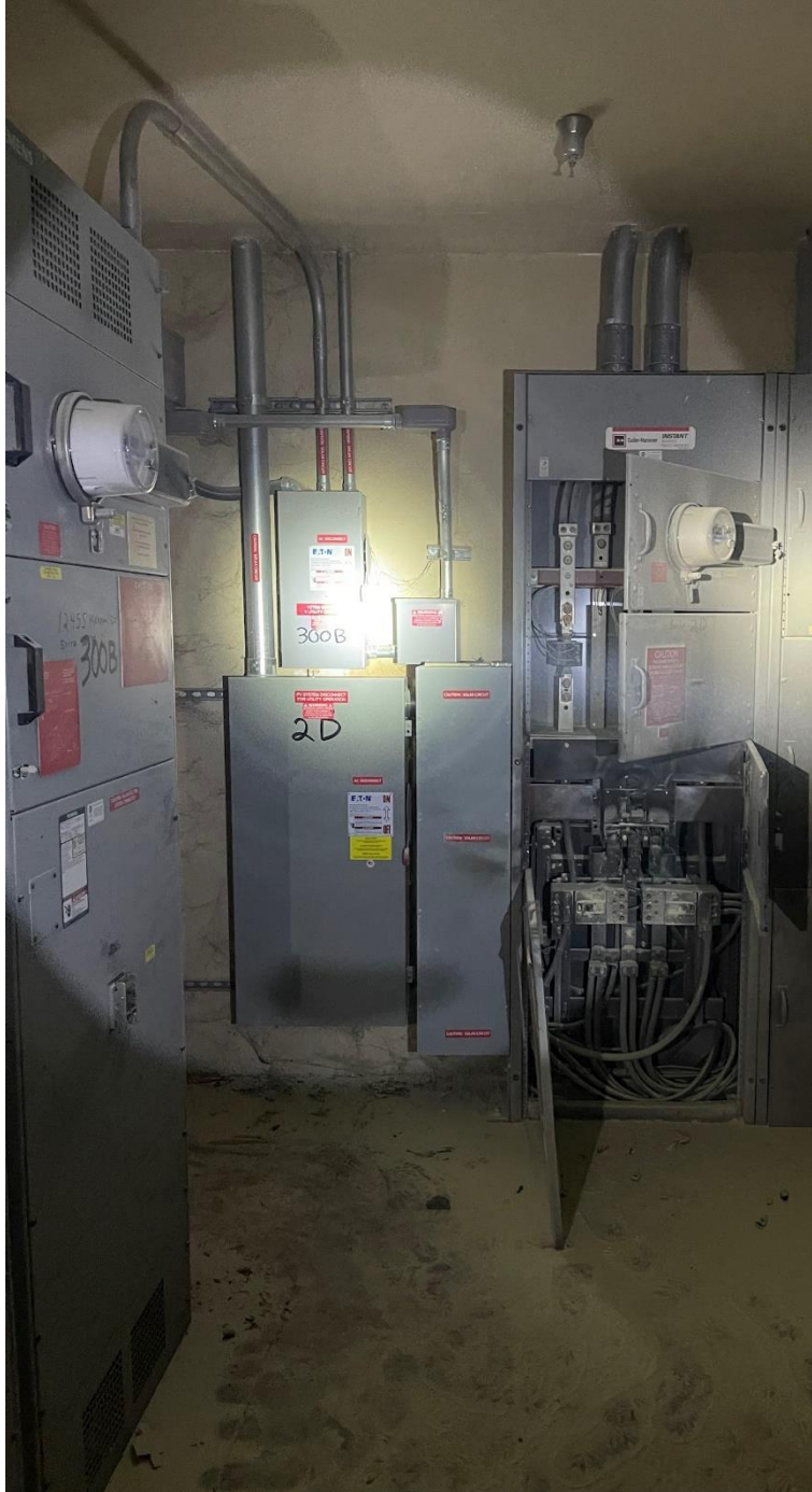
Image 7 - Electrical Room (Interior), Damaged Electrical Panel
