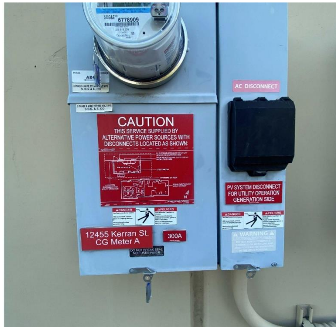
Image 5 - Solar (PV) Meter
