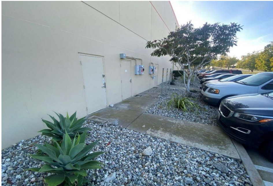
Image 3 - Electrical Room Entrance (Alpha Side of Structure)
