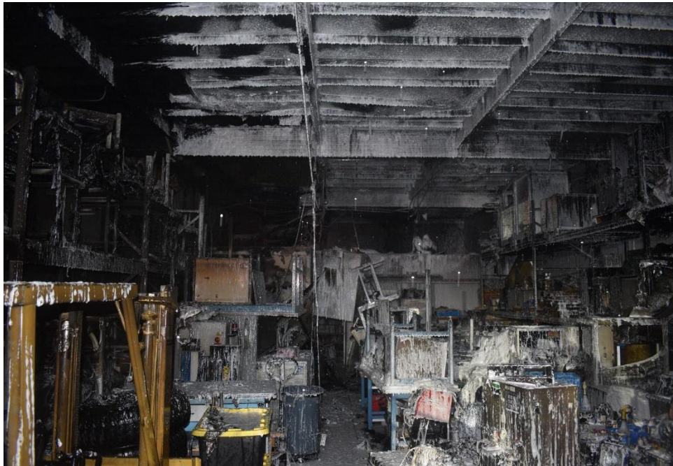
Fire Result, damage
